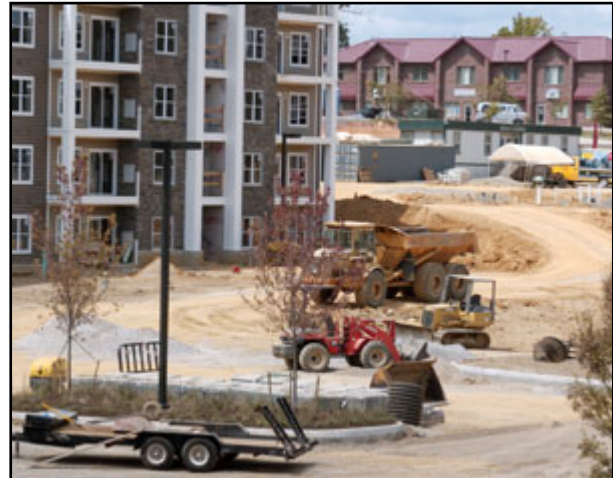
Smith's Landing in Blacksburg – a construction site visited by students during the spring 2008 offering of Advanced Land Development Design. Course instructors from Draper Aden Associates provided site engineering services on the project.
